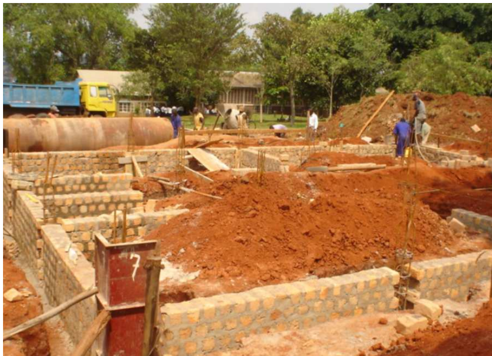
Fig 3: Construction work at Computer Refurbishment centre as of 15/06/07 (More about the Computer Refurbishment centre is contained the Permanent Secretary statement – Appendix 2).
